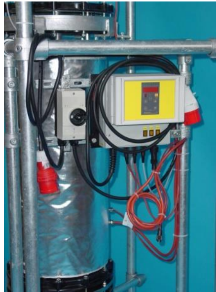
Elektr. Heizung/ Electrical heating
