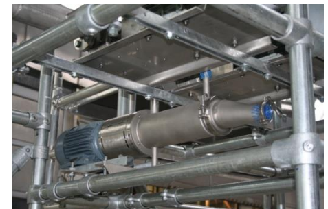
Misch-Pumpe/ Mixing pump
