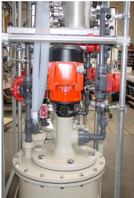
NaOH-Vorlage m. Uml.-Pumpe/ NaOH-Tank with circulat. pump
