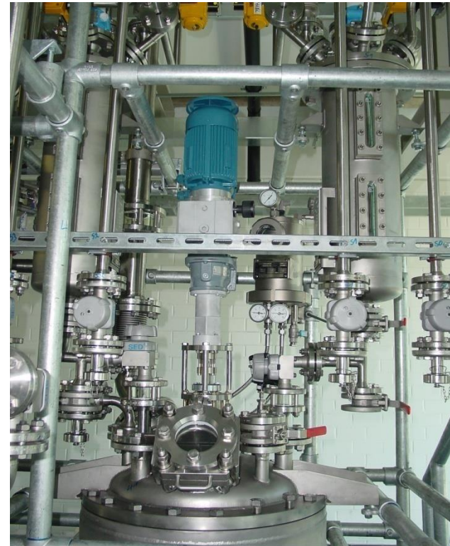
Rührbehälter - Detail / Mixing vessel - detail
